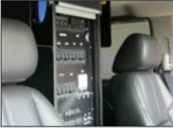
Electrical system control panel in front cabin
